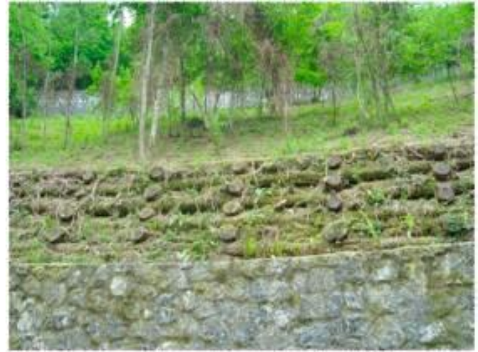
slope crib wall at Desiata, Seravezza (LU), with similar willow cuttings original density
