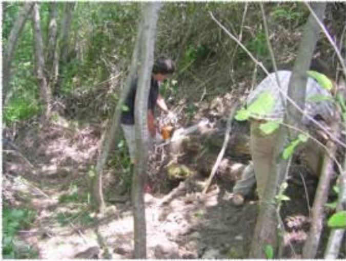
bank crib wall at Molino di Lierna, Poppi (AR), with initial 10 willow cuttings per square meter and to date alder natural renewal
